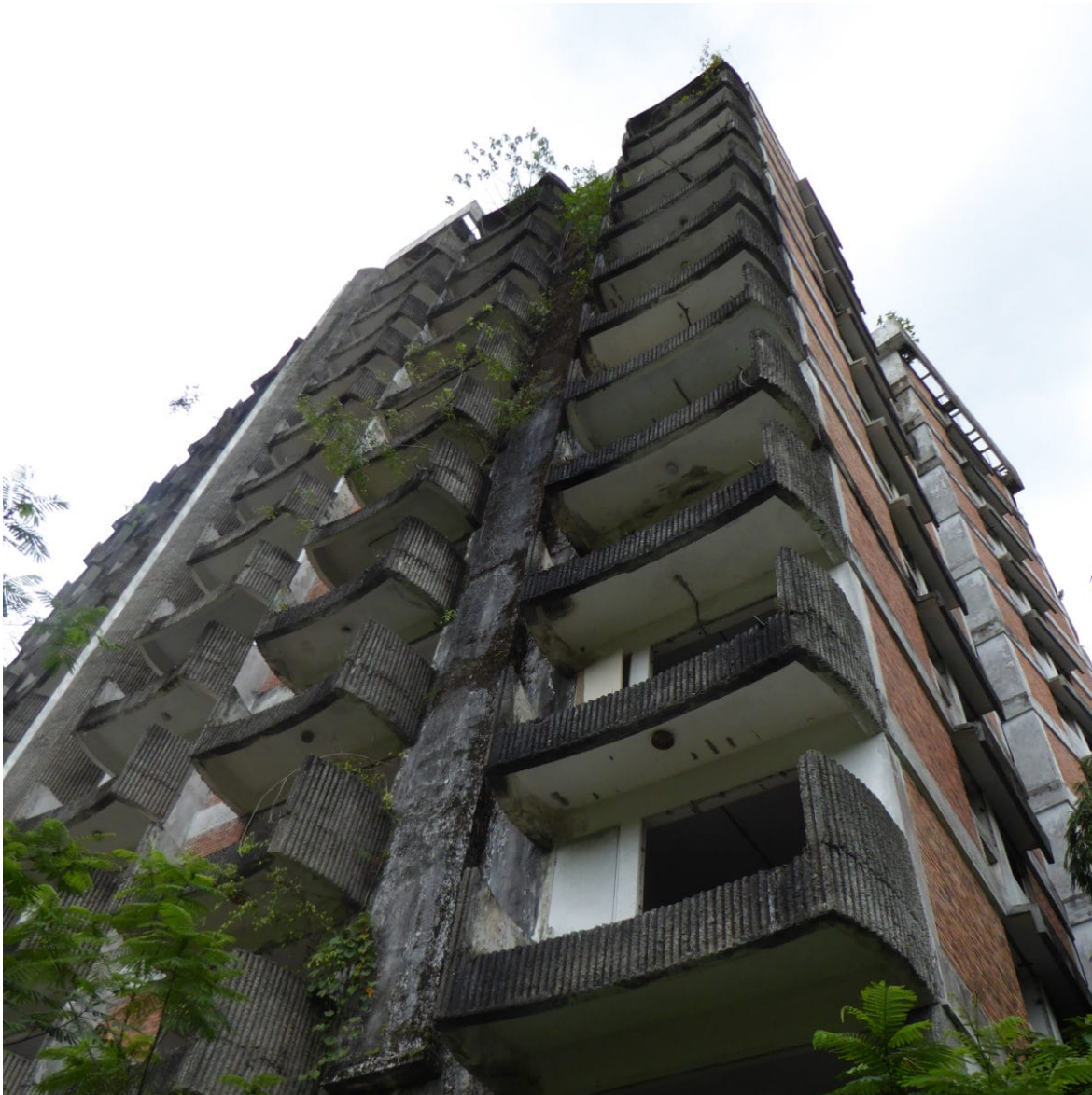
Highland Towers, Malaysia © Veronika Fendel
